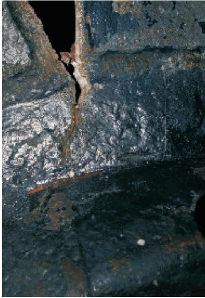
Figure 6. The crack initiation and branching of the crack on the bottom close to the peripheral weld (connecting the bottom dome with the lower support ring frame)
